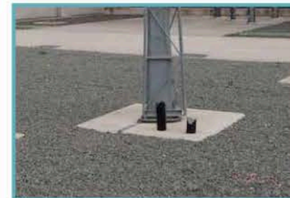
Plate 73 - Concrete pads to base of electrical equipment
