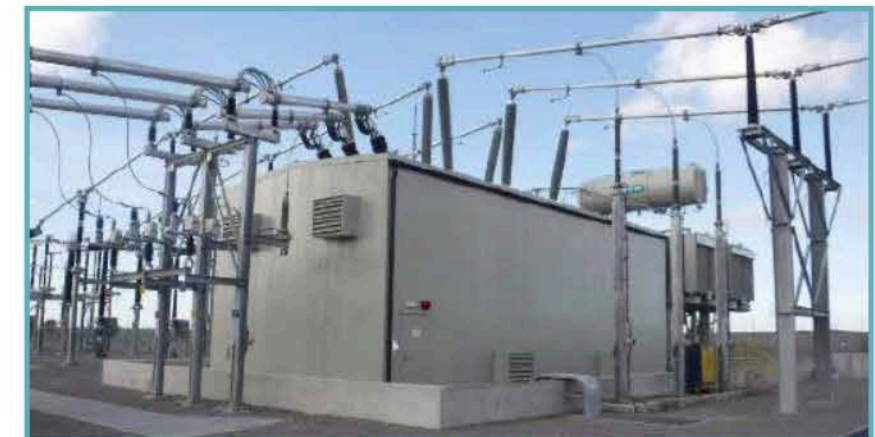
Plate 64 - Transformer with noise enclosure (source - RWE)
