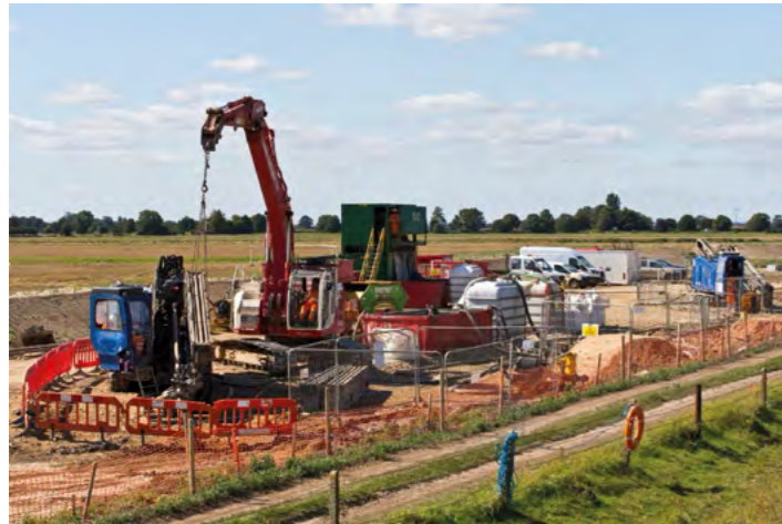
Indicative image of a HDD site. Image courtesy of RWE from the construction of Triton Knoll Offshore Wind Farm, Lincolnshire. North Falls Offshore Wind Farm's construction may differ.
