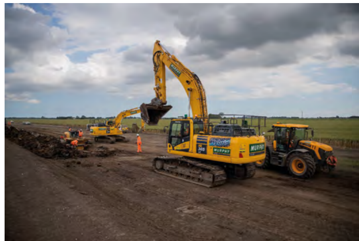
Indicative image of temporary construction haul road construction. Image courtesy of RWE from the construction of Triton Knoll Offshore Wind Farm, Lincolnshire. North Falls Offshore Wind Farm's construction may differ.
